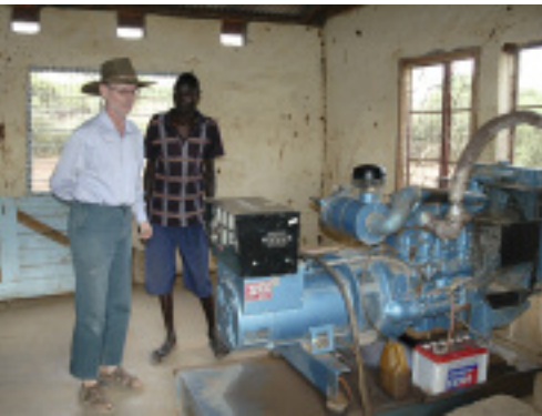
Pumpstation in Barpello/Kenia.
